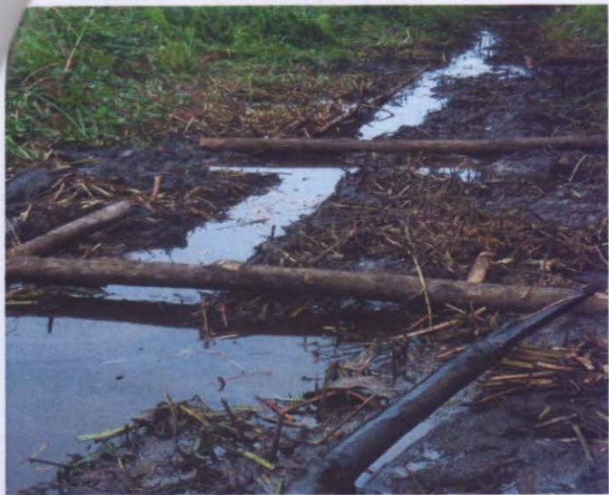
Figure 1: Cut and Harvested Flowline
