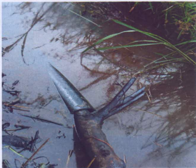
Figure 2: Cut and Harvested Flowline
